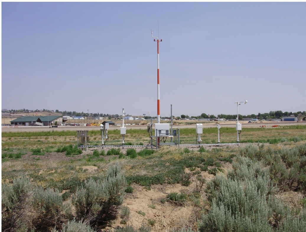
The Automated Surface Observing System (ASOS) at the Elko Regional Airport currently produces the official weather observations for Elko. Photo by author.
