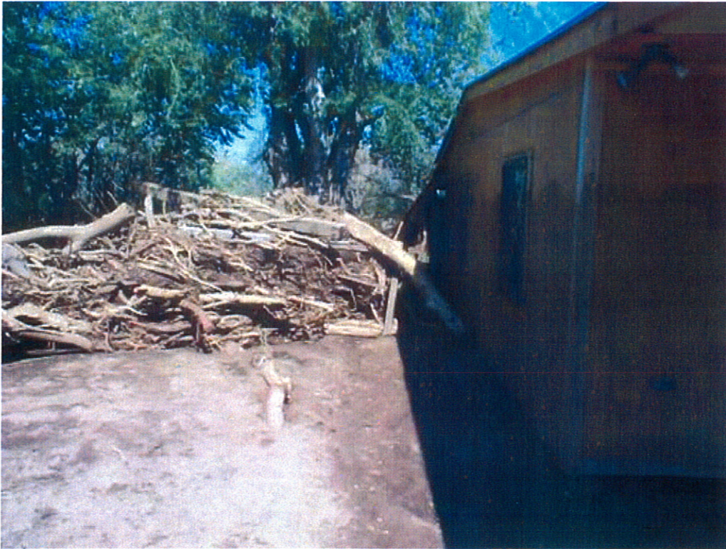
Figure 6. Large pile of debris near channel side of residence. Note highwater mark along side of residence.
