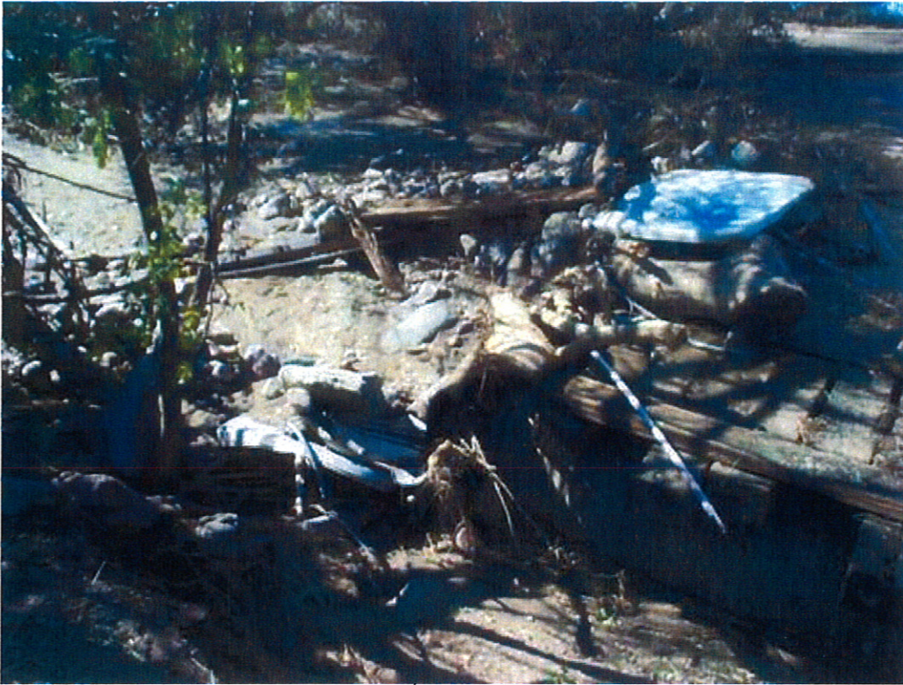
Figure 7. Culvert and wooden beam bridge 100 yards downstream of residence. Note culverts blocked and channel deposition upstream.
