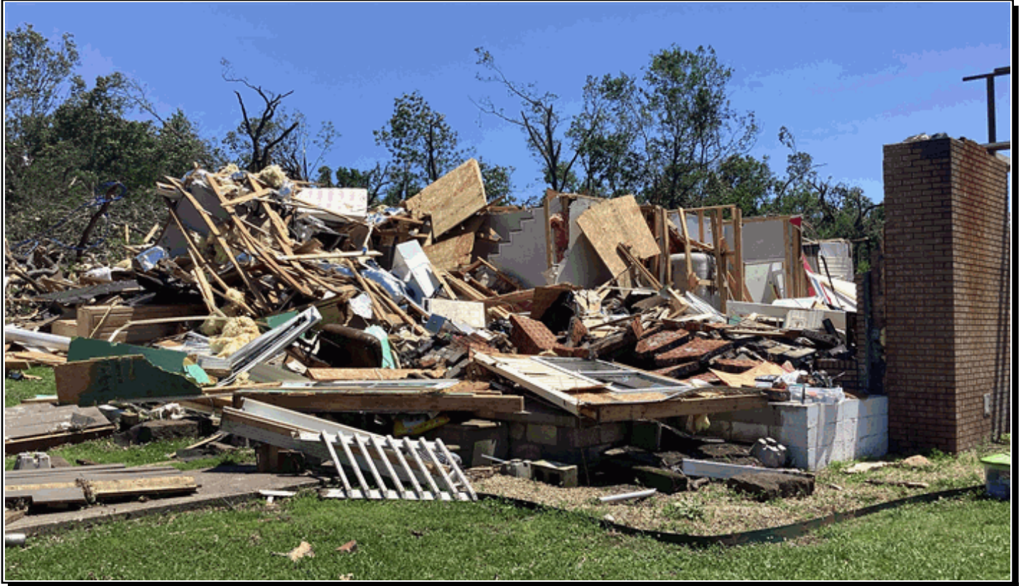
An EF-3 tornado destroyed more than 70 homes and businesses, and damaged at least 1200 others, in Rogers and Mayes Counties, during the late evening of May 25, 2024. Two people were killed by the tornado, and at least 23 others were injured. Damage to trees and power poles was extensive. Photo by Ed Callanese, WCM, NWS Tulsa Oklahoma.
