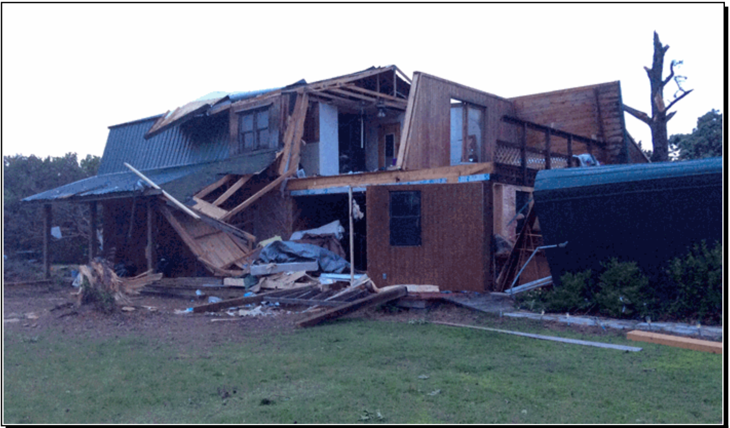
An EF-2 tornado severely damaged homes, destroyed numerous barns and outbuildings, and partially collapsed a cell phone tower near Poteau, Oklahoma, on the evening of May 25, 2015. Photo by Ed Calianese, WCM, NWS Tulsa Oklahoma.
