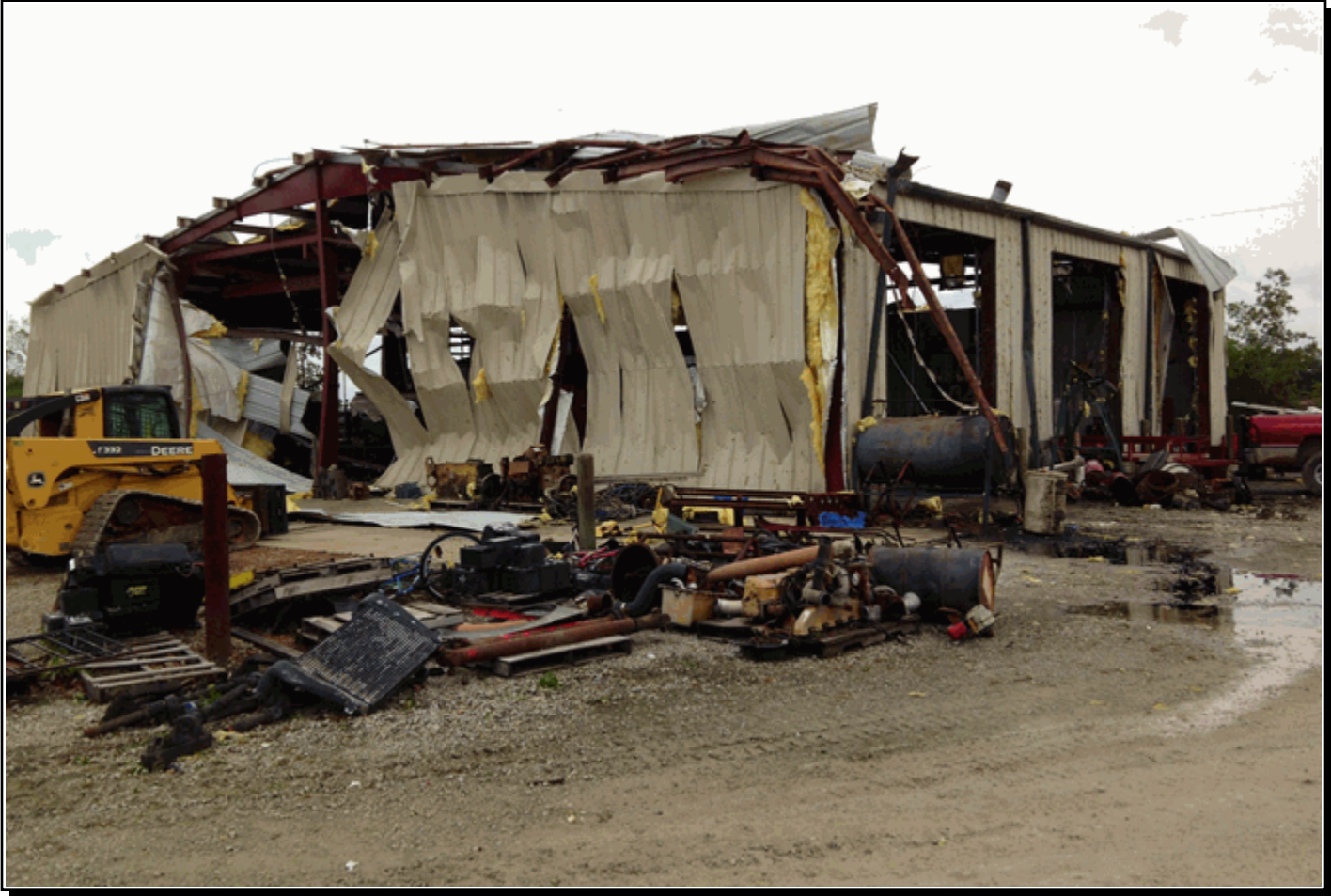
An EF2 tornado severely damaged a metal building northwest of Wyandotte in Ottawa County, Oklahoma, during the evening hours of May 20, 2013. Photo by Ed Calianese, WCM, WFO Tulsa.
