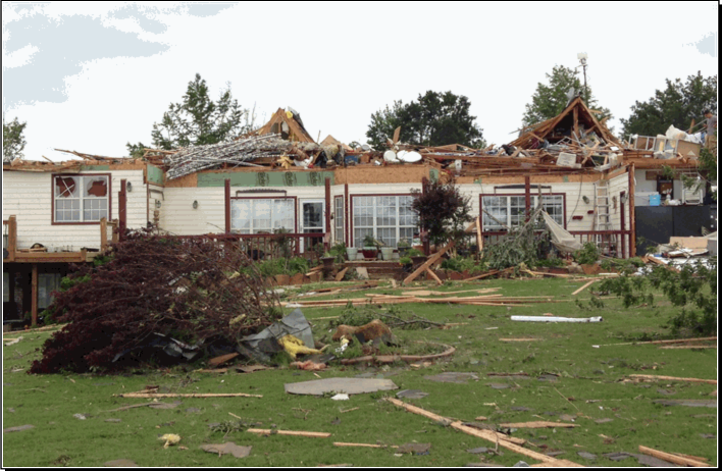
An EF2 tornado severely damaged a house in Broken Arrow in Wagoner County, Oklahoma, during the evening of May 30, 2013. Photo by Ed Calianese, WCM, WFO Tulsa.
