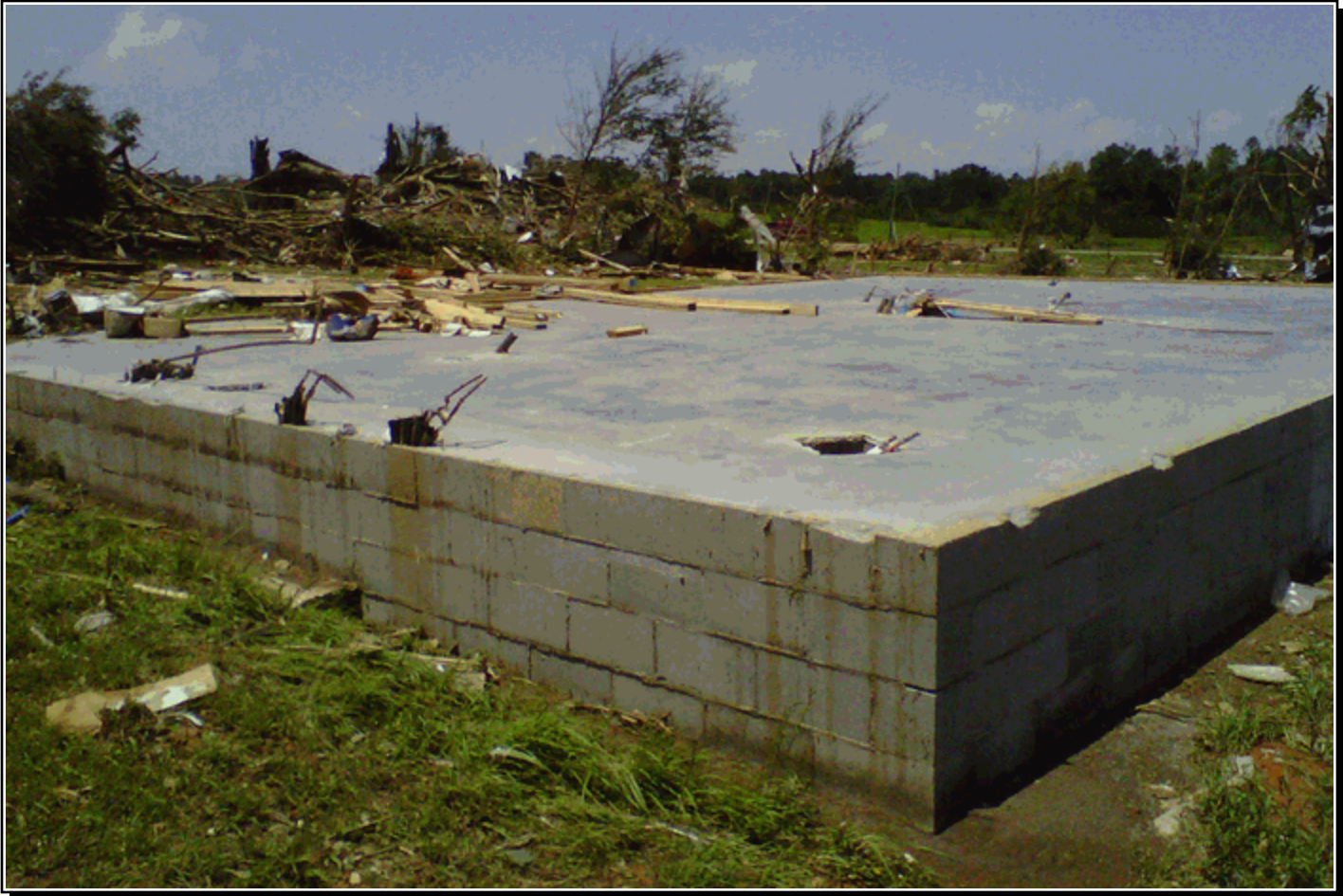
An EF-4 tornado destroyed this home as well as a number of others in the Etna area of Franklin County, Arkansas, on the evening of May 24, 2011. This tornado ultimately killed four people in Franklin and Johnson Counties. Photo by Ed Calianese, WCM, NWS Tulsa Oklahoma.
