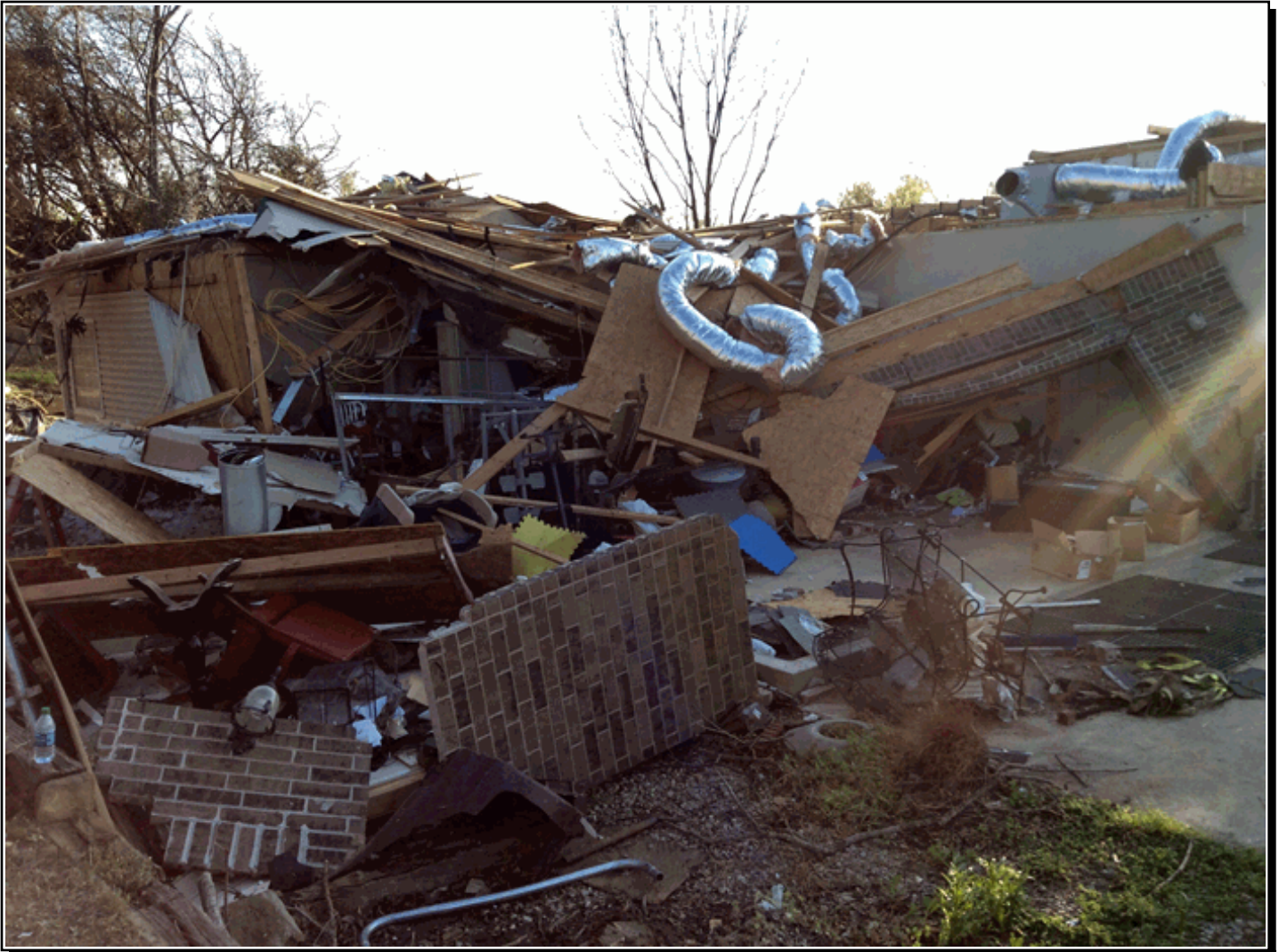
An EF-2 tornado severely damaged homes, destroyed barns and outbuildings, and snapped numerous trees and power poles near Claremore, Oklahoma, on the evening of March 30, 2016. Photo by Ed Calianese, WCM, NWS Tulsa Oklahoma.
