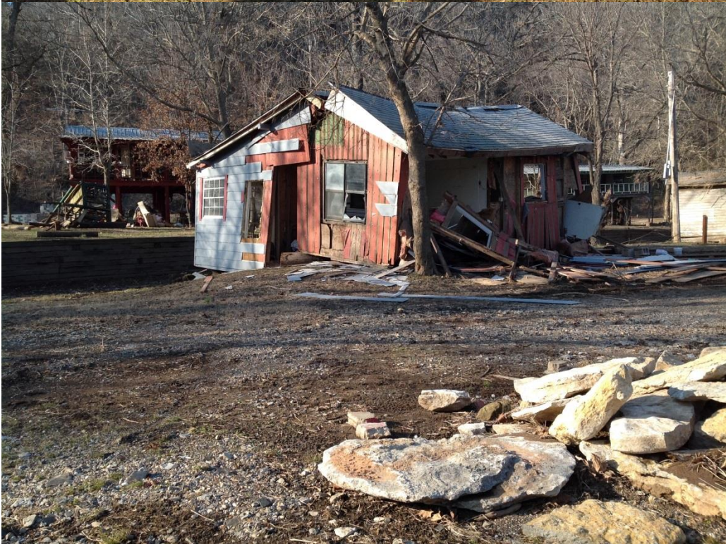
Fig. 21. Illinois River flood damage at Spencer Ridge/Fidlers Bend area. Displaced cabins. (image: Nicole McGavock, NWS Tulsa)
