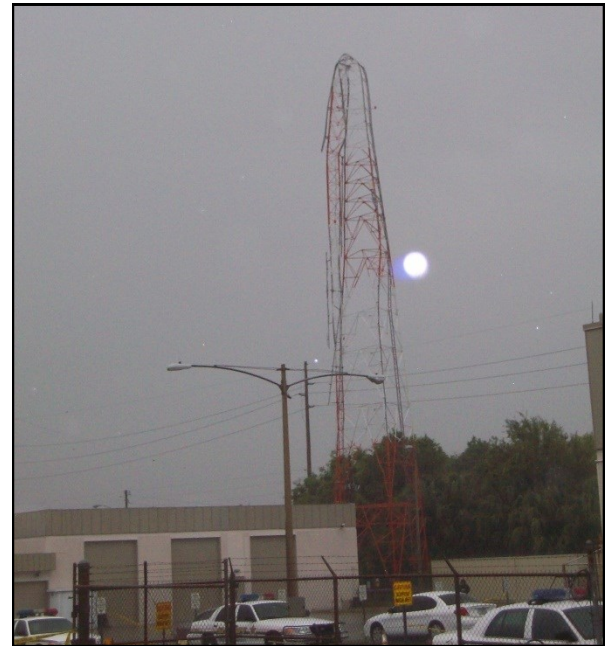
Tower collapse at Position 3. Winds near the ground estimated at 60 MPH while winds at top of tower estimated at over 110 MPH.
