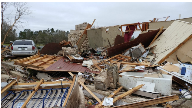
Home with EF-3 damage at the strongest point of the Leon/Jefferson County, FL tornado.
