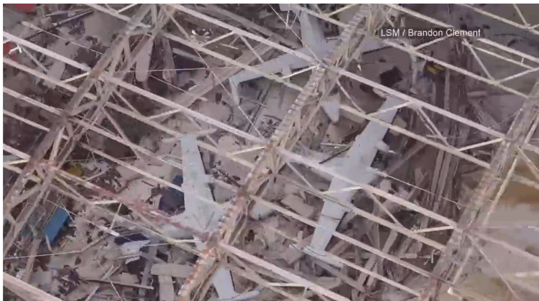
Figure 13: Catastrophic damage at Tyndall Air Force Base with fighter jets exposed inside of roofless hangars (Source: First Coast News -- www.firstcoastnews.com )
