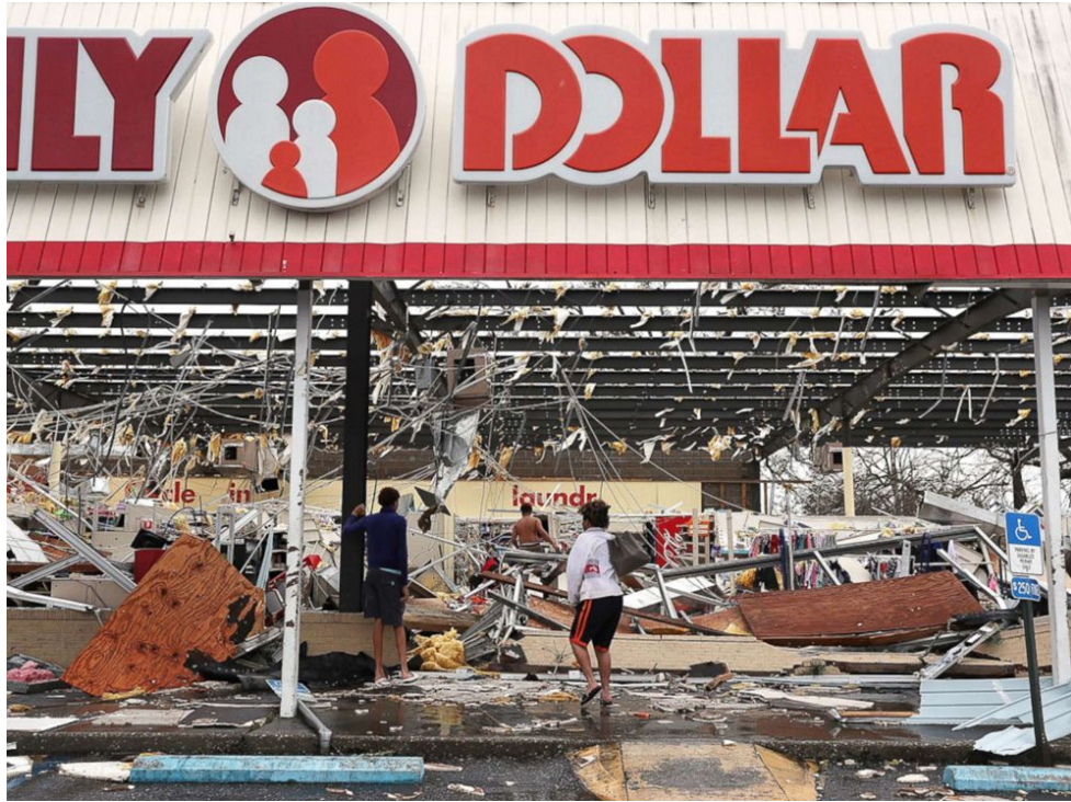
Figure 14: Family Dollar damaged by hurricane Michael (Source: First Coast News -- https://www.circa.com/story/2018/10/11/nation/family-dollar-looted-in-the-aftermath-of-hurricane-michael/ )
