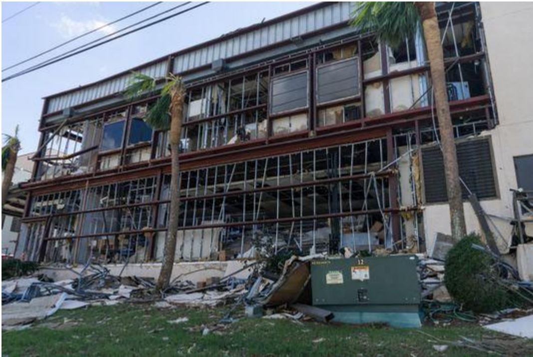
Figure 12: Bay Medical Center Sacred Heart: The hospital sustained roof, structural and water damage (Source: Pensacola News Journal -- www.pnj.com/news/ )
