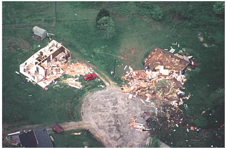
(Photograph courtesy of Tim Marshall, Structural Engineer, Haag Engineering, Dallas, TX)
