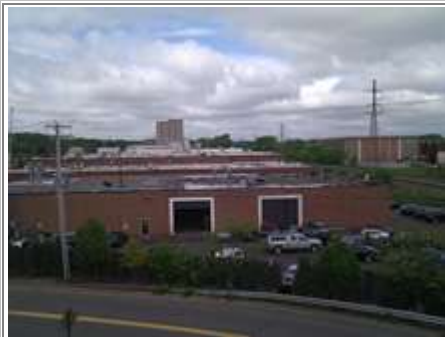
Roof Damage to a business in St Louis Park, MN
