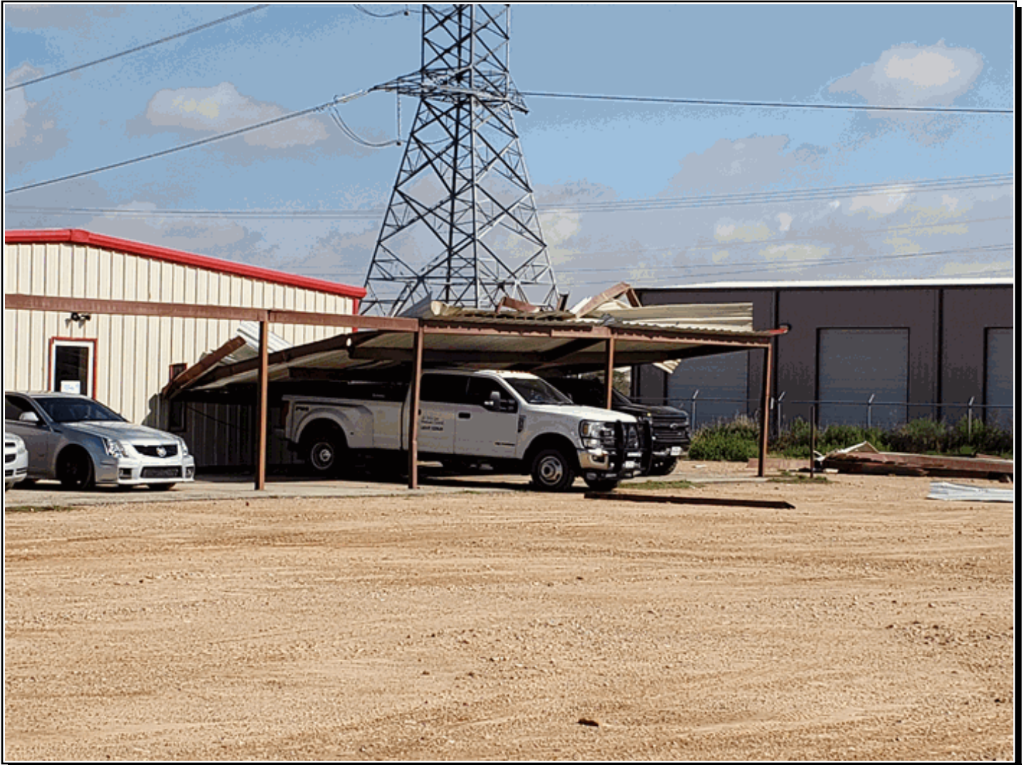
A thunderstorm moved across Midland County and produced wind damage in Greenwood. A carport collapsed. Picture is courtesy of Charles Yaws.
