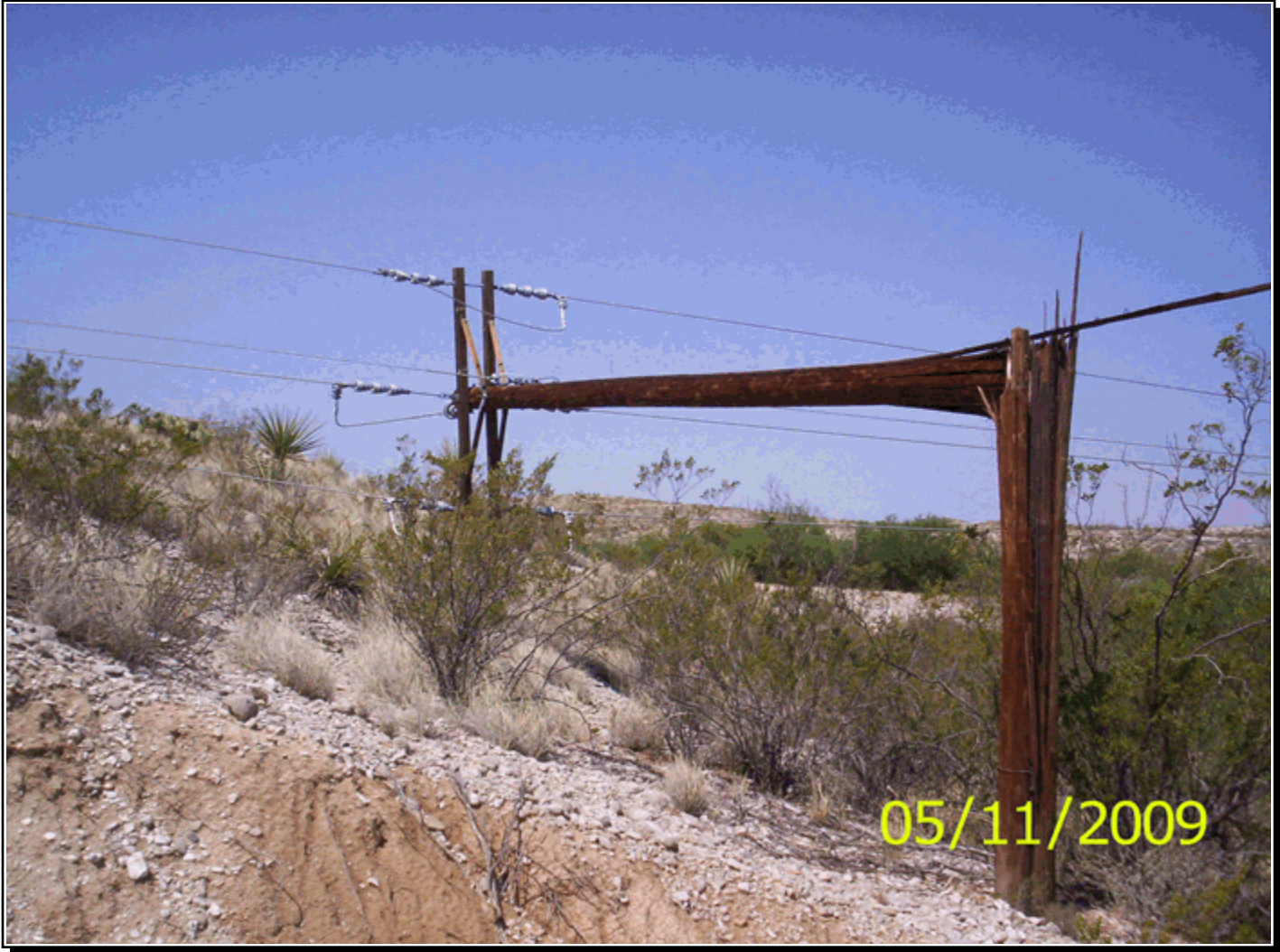
Image showing a power pole snapped near its base along the damage path. This photo was taken by Pat Vesper, WCM WFO Midland, TX.
