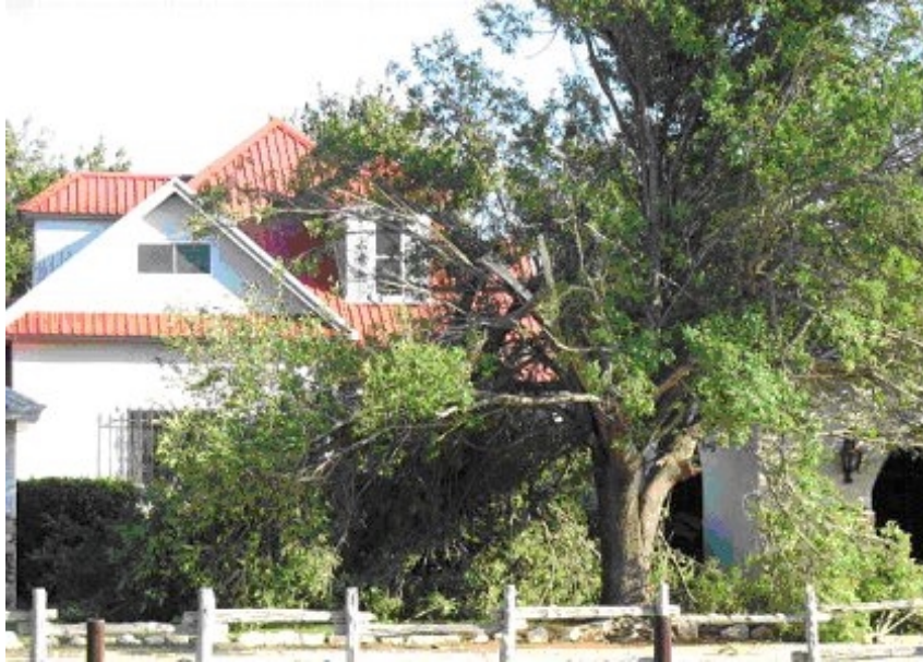
A tree was split by severe thunderstorm winds in Andrews. Photo Courtesy: Mike Cook - Andrews County Emergency Manager
