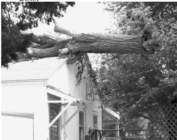
A tree was blown onto this house in Seagraves by 75 mph wind gusts. Photo courtesy: Tri County Tribune (Seagraves, Texas) photo/P. Christine Mills
