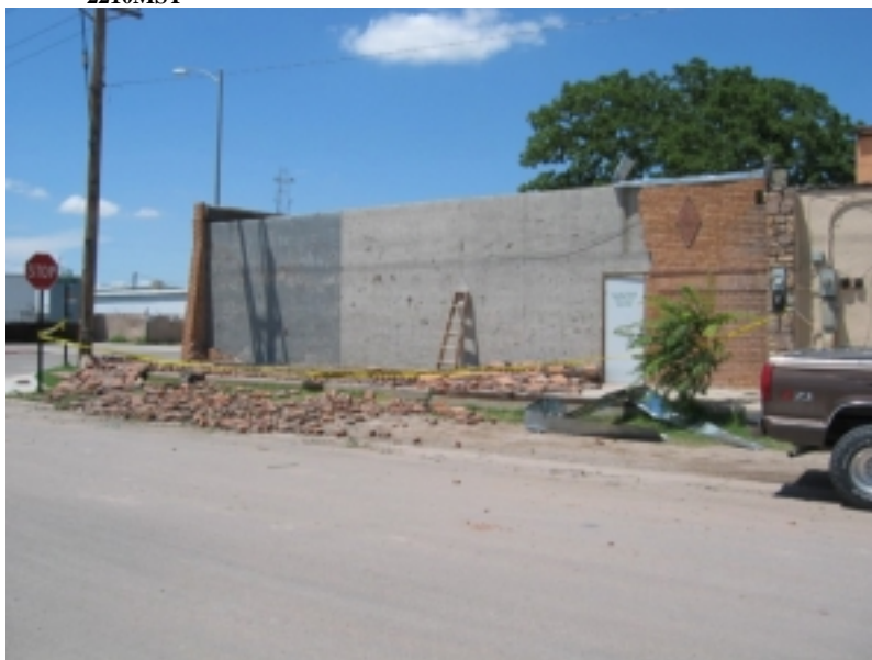
Damaging thunderstorm winds affected a large part of Eddy County on the evening of the 12th. Downed power lines, poles, and trees were widespread in the area between Carlsbad and Malaga. Numerous light structures also were damaged. The photo above shows an exterior brick wall that collapsed when a portion of the roof was peeled off of a Malaga business by the winds. Photo courtesy: National Weather Service Midland/Odessa, Texas.
