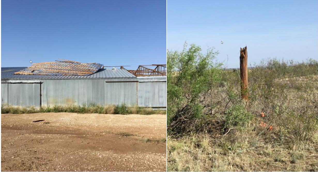
Metal roof of a large barn in Belding blown off due to the winds from the storm (Left Image). One of many snapped power poles along Old Alpine Hwy, FM 2057 due to the strong winds (Right Image).
