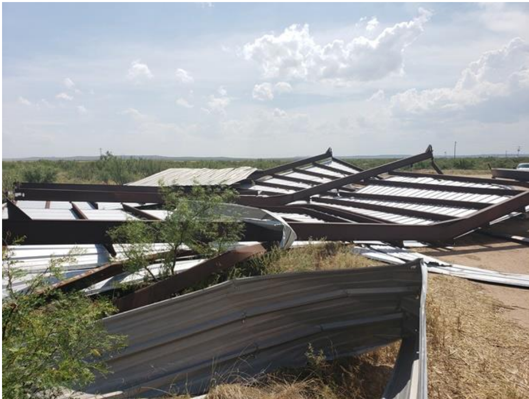
Hay Barn in Belding, TX that completely collapsed due to the severe winds from the storm
