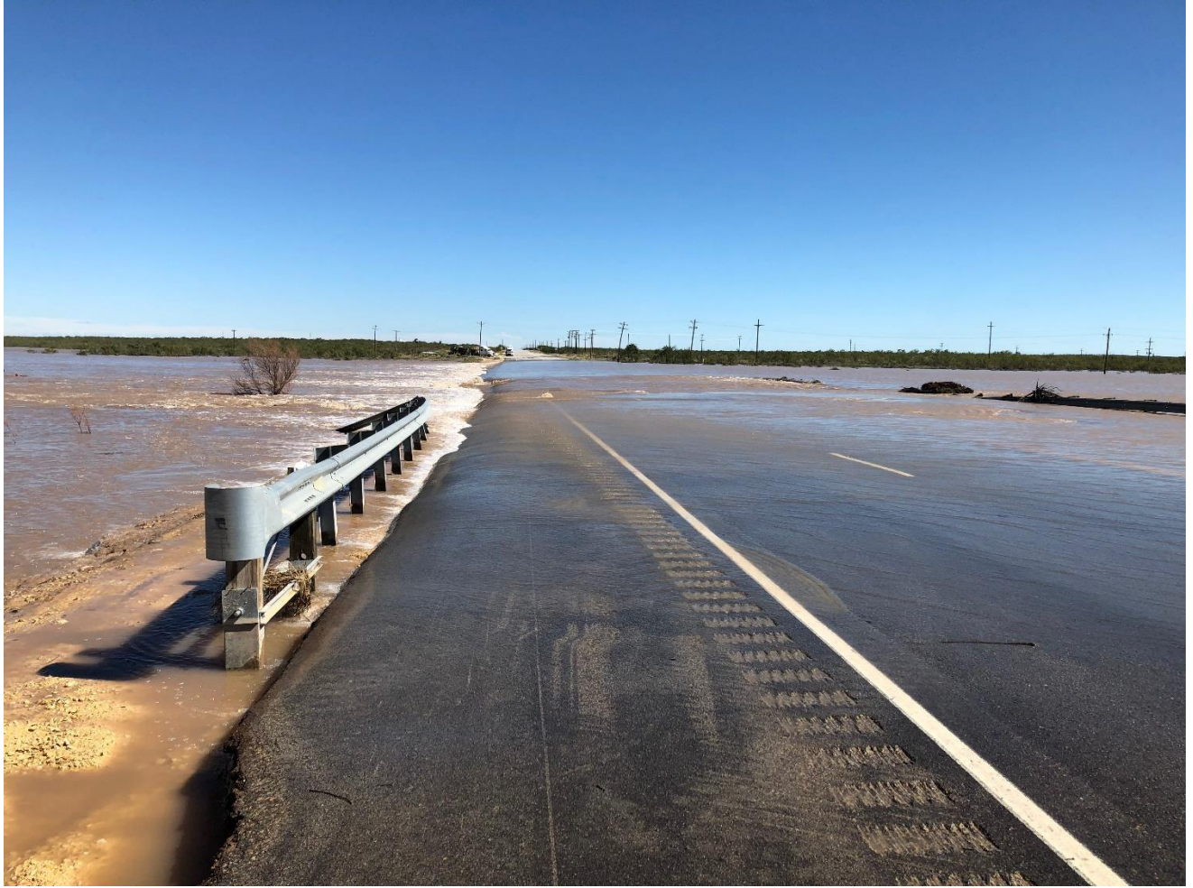
Figure 9 – Flooding along TX 158 between Midland and Garden City, Texas.
