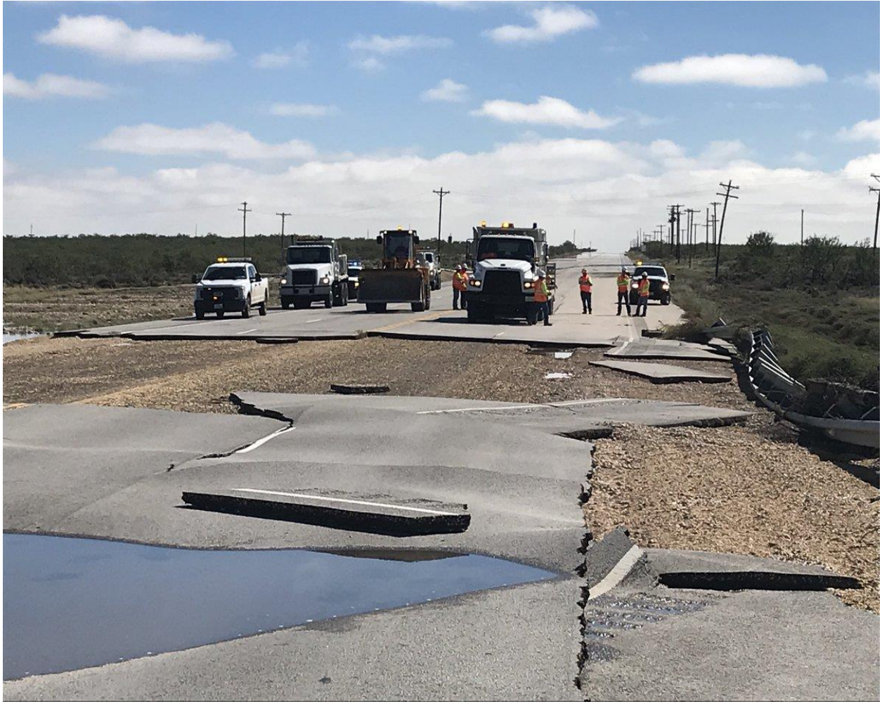
Figure 5 – Major Road Damage between Midland and Garden City, Texas on TX 158.
