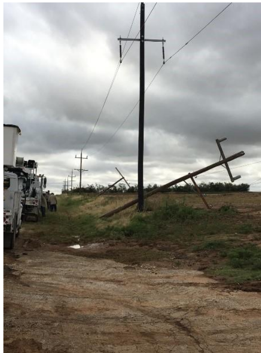
Figure 14 – Power pole damage along Interstate 20 near mile marker 224 in Mitchell County, Texas.
