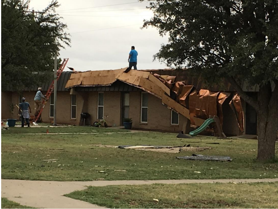
Figure 11 – Dorm at Midland College with its roof damaged.
