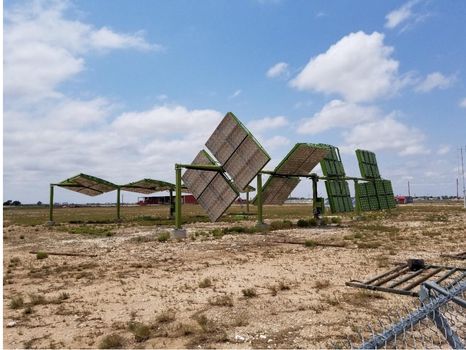
Figure 7 – Damage to solar panels at New Mexico Junior College in Hobbs, New Mexico.
