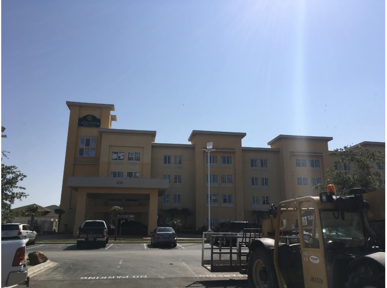
Figure 9 – Broken windows from hail at the La Quinta hotel near Faudree Road and Highway 191 in Odessa, Texas.
