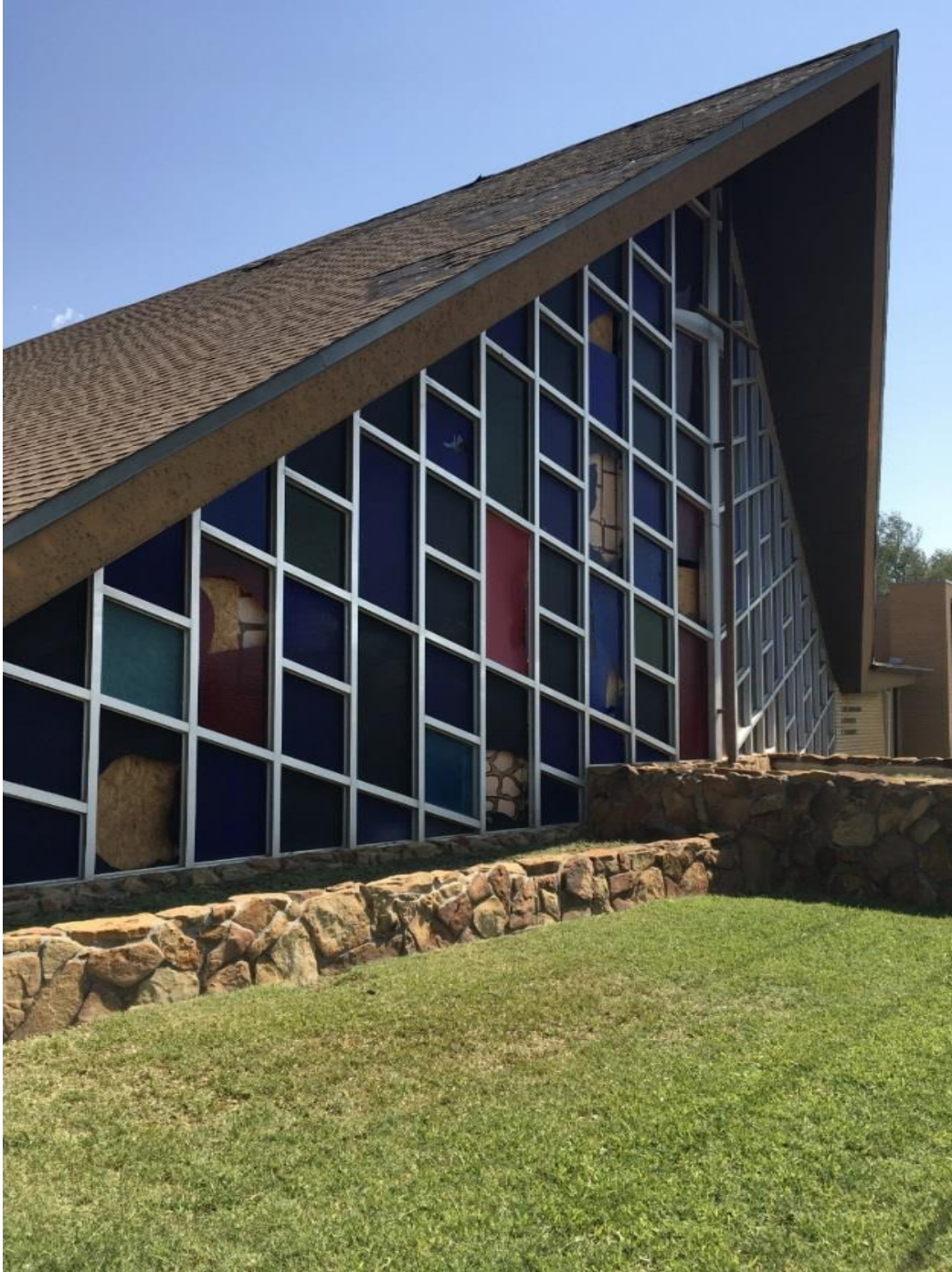
Figure 13 – Hail damage at Sherwood Baptist Church near E 42 nd Street in central Odessa, Texas.
