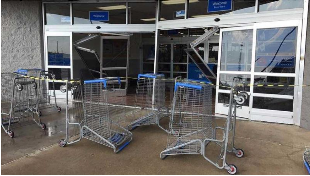
Figure 6 – Wind damage to front doors at Walmart in Odessa, Texas (Courtesy of Daniel Carnes).
