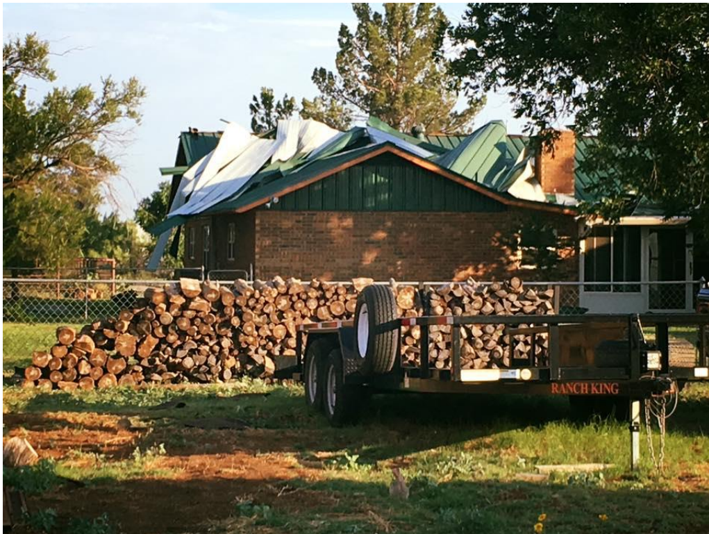
Figure 5 – Metal roof damage in West Odessa, Texas (Courtesy of Judy Woolf).
