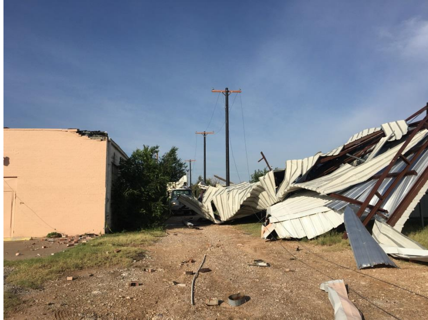
Figure 6 – Wind damage (Courtesy of Amber Hluchan).
