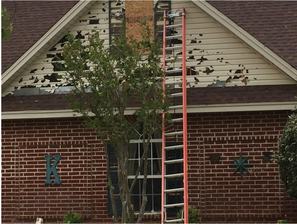
Figure 6 – Hail damage in the west part of Seminole, Texas (Courtesy of Mark Strobin).
