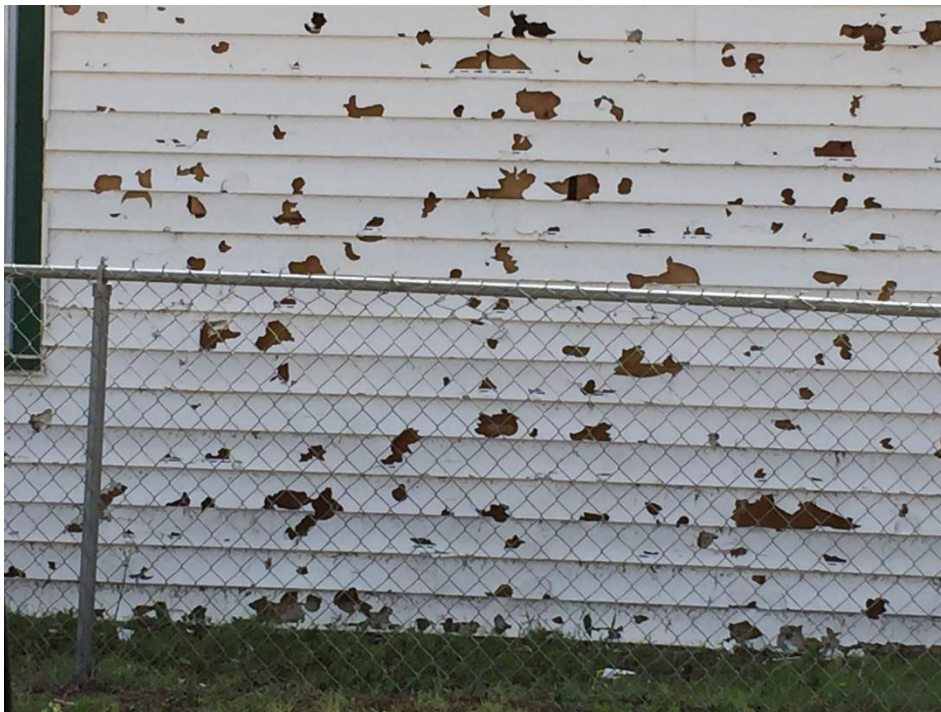
Figure 7 – Hail damage in the west part of Seminole, Texas (Courtesy of Mark Strobin).
