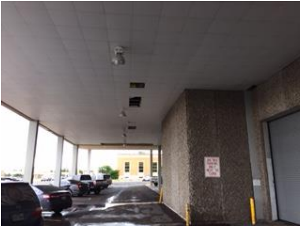
Figure 6: Ector County, Texas Courthouse with missing ceiling tiles.
