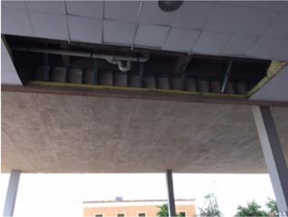
Figure 5: Ector County, Texas Courthouse with missing ceiling tiles.
