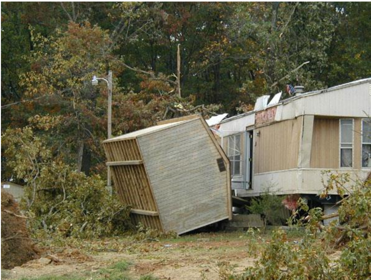
Close-up of unanchored shed rolled into a mobile home and some snapped trees in the Country Star Mobile Home Community.
