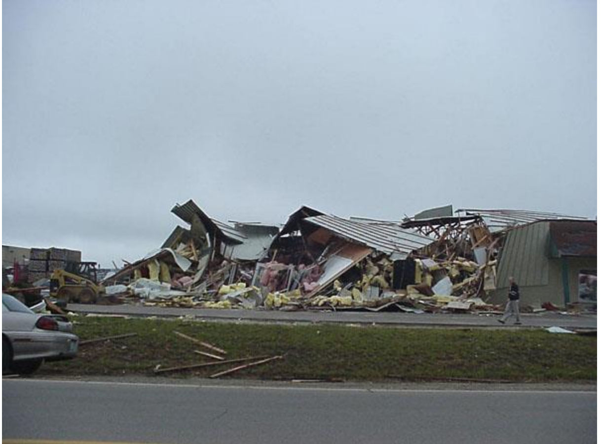
Total view of the first building. Viewing west. The tornado approached the lumberyard from the west.
