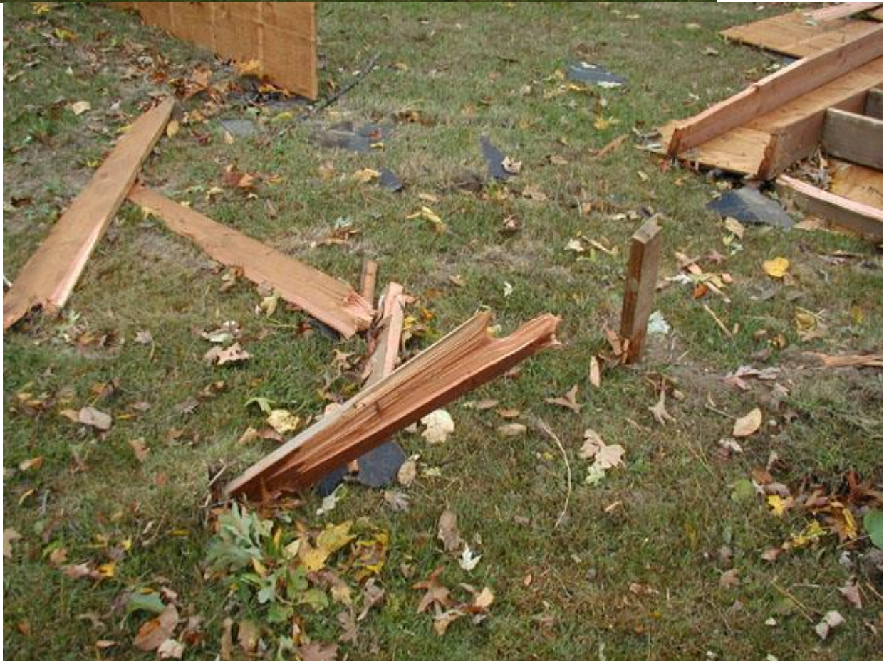
Missiles (pieces of debris) originating from the Iron County Health Center roof driven into the ground around 75 yards away on the north side of Russell Street.
