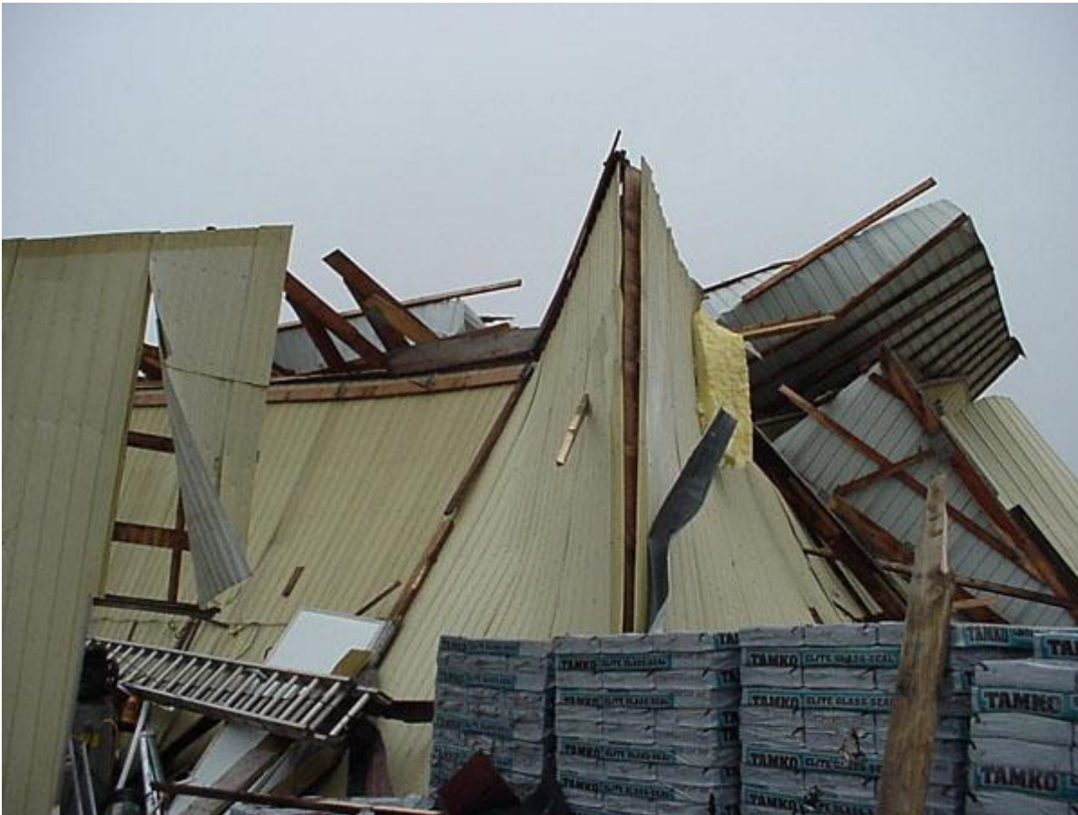
Example of missiles embedded within the sheet metal associated with the first building.
