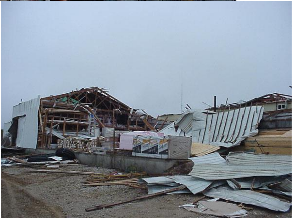
Damage to a third building near the western part of the lumberyard. Part of this building was totally destroyed. Viewing north-northeast.
