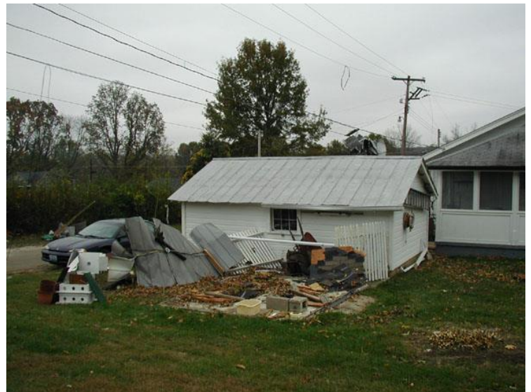
A south view from the rear of a house at the corner of Wayne and Russell Streets in Ironton. Note remnants of the metal shed in the power lines behind the house and its original location in the foreground of the picture.
