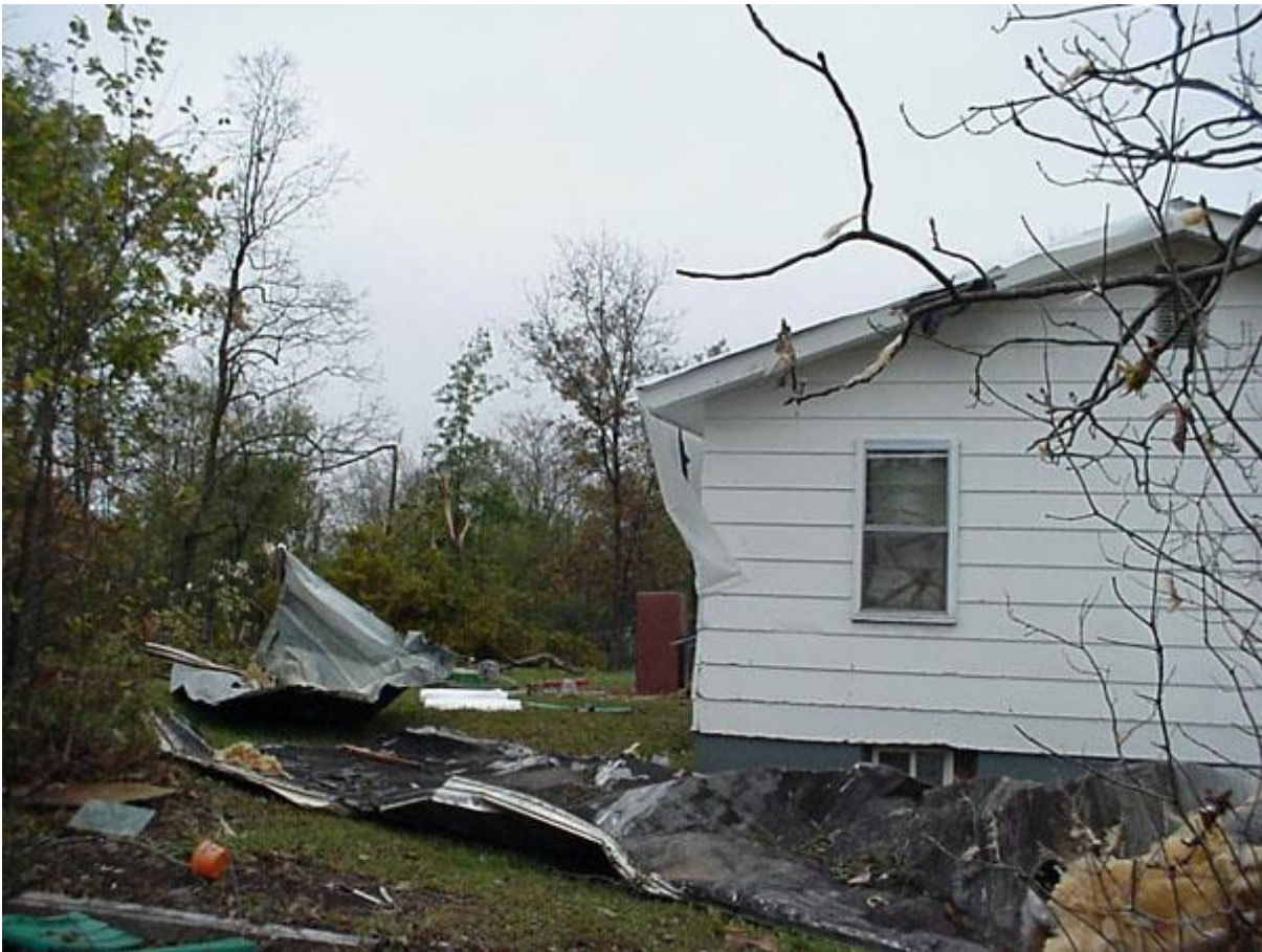
Another view of the home damage along the east side of East State Highway caused by the second of five tornadoes.
