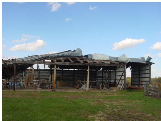
(Tornado #3 - north of Paris, MO) Machine shed near the southern part of the third tornadic damage track. (Viewing north-northeast).
