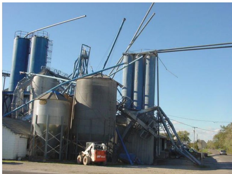
The grain-bin storage facilities including the cat walk was damaged in Calwood, Missouri. (Viewing north)
