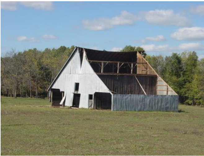
(Tornado #1) Roof of a barn damaged and tossed to the northeast some 50 to 100 yards. The barn was located on the north side of County Road 943. (Viewing northwest).
