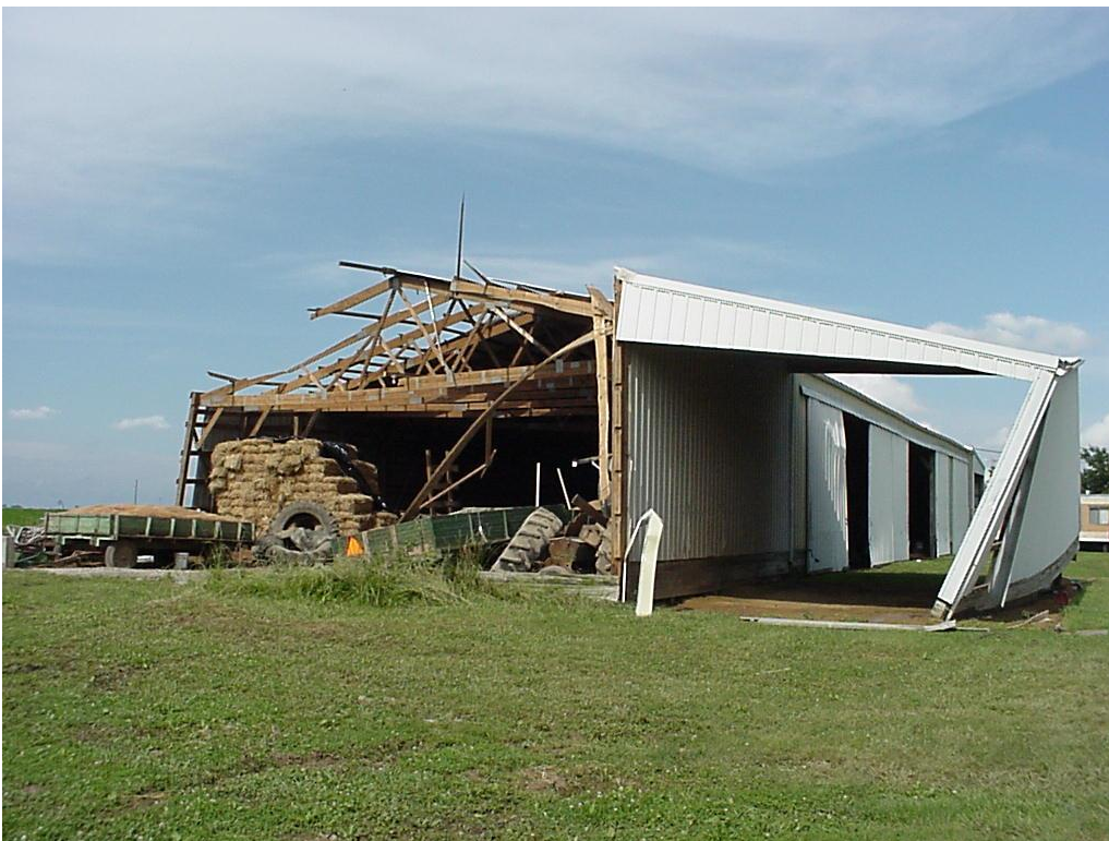
Damage to a machine shed on the west side of a farmstead 2.2 miles west of Plum Hill, Illinois just south of Highway 15
