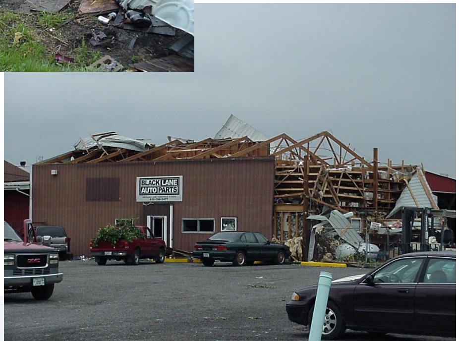
Roof of a large machine shed located on the east side of Black Lane severely damaged (Caseyville, IL)
