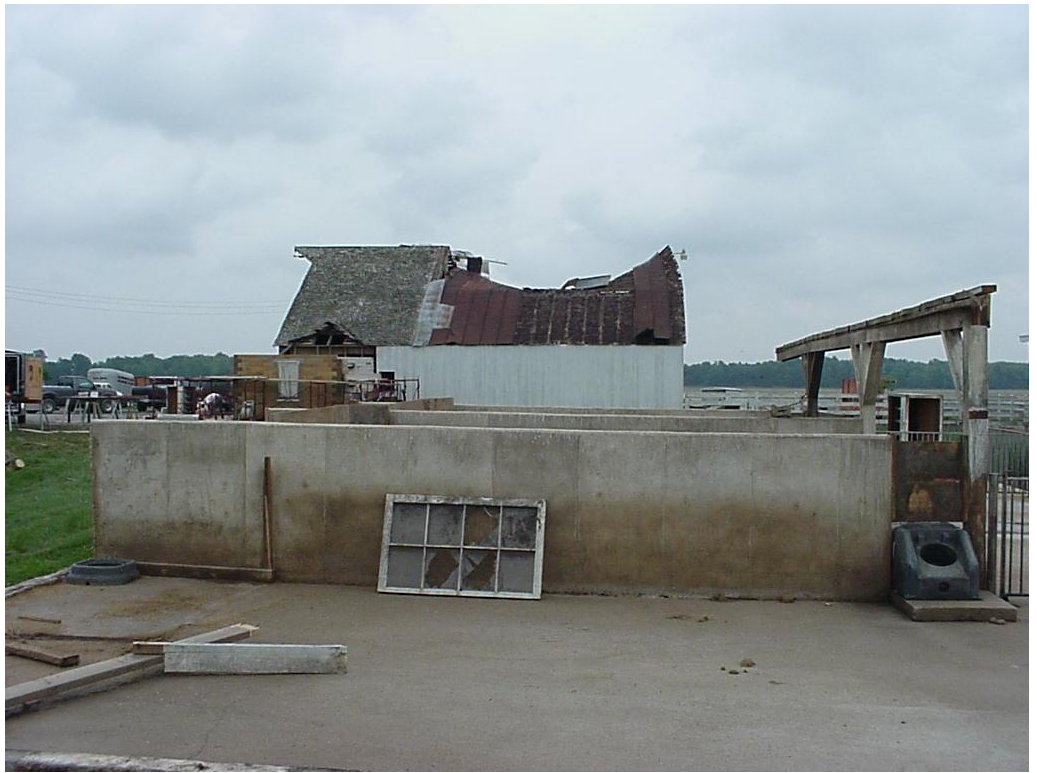
Damage to a barn and hog barn on the farmstead 4 miles south of Germantown (Clinton County, Illinois)
