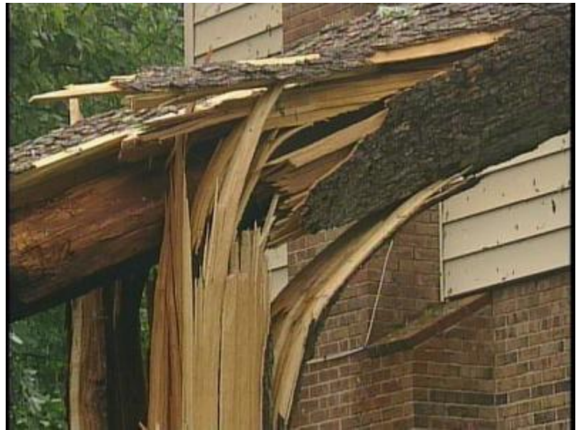
Tree blown down onto a house. Photo courtesy of KSDK Channel 5.
