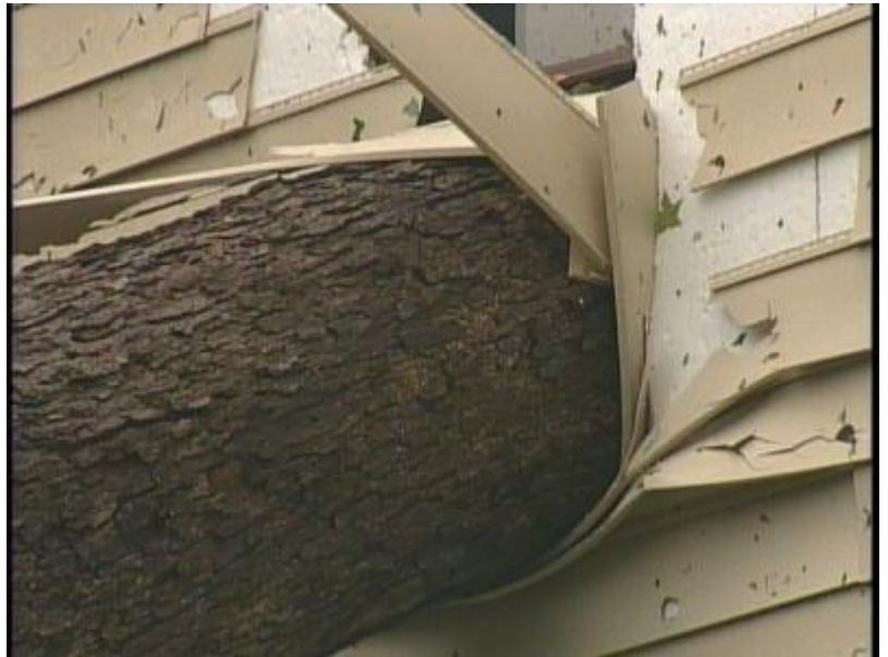
Another picture of tree that fell onto a house. Photo courtesy of KSDK Channel 5.
