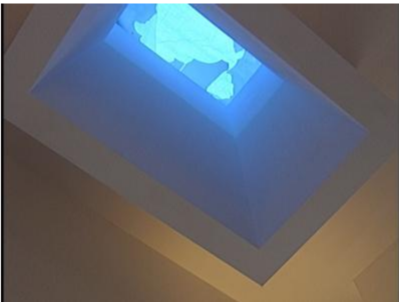
Broken skylight due to large hail. Photo courtesy of KSDK Channel 5.
