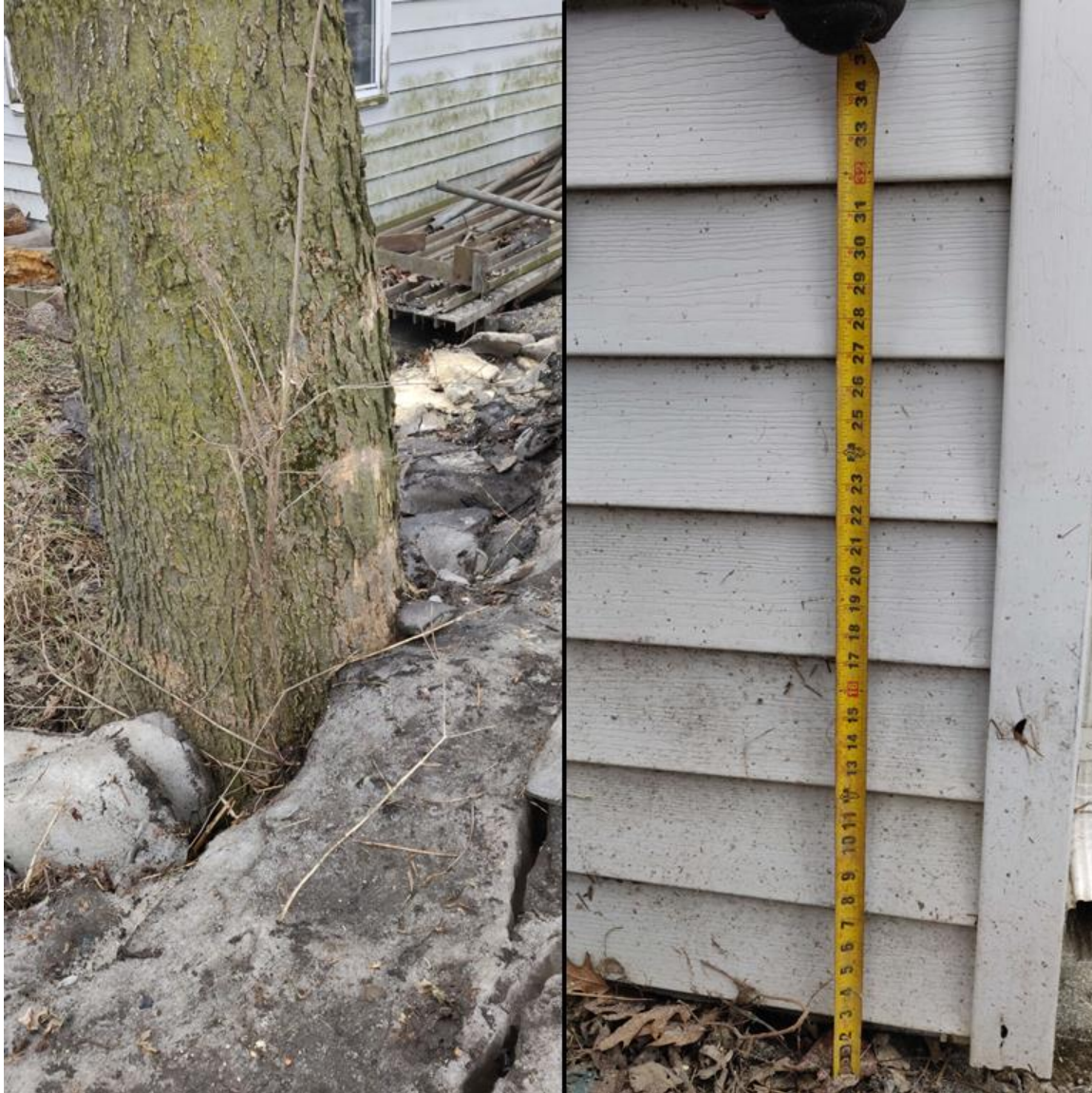
Figure 19. Damage marks to a tree and debris marks on a garage approximately 2 miles downstream of Wilmington remain visible on February 6. These high water marks suggest a peak water level of about 531.5 feet elevation.
