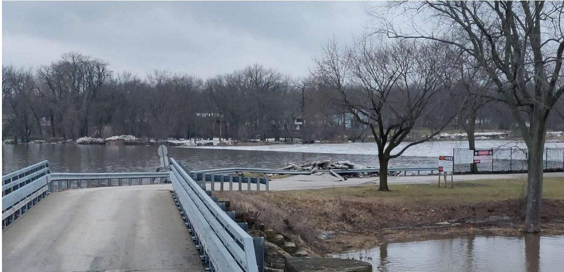
Figure 11. Damage to the roadway through Island Park in Wilmington. Note the piles of ice and shear walls on the opposite river bank still visible on January 30.
