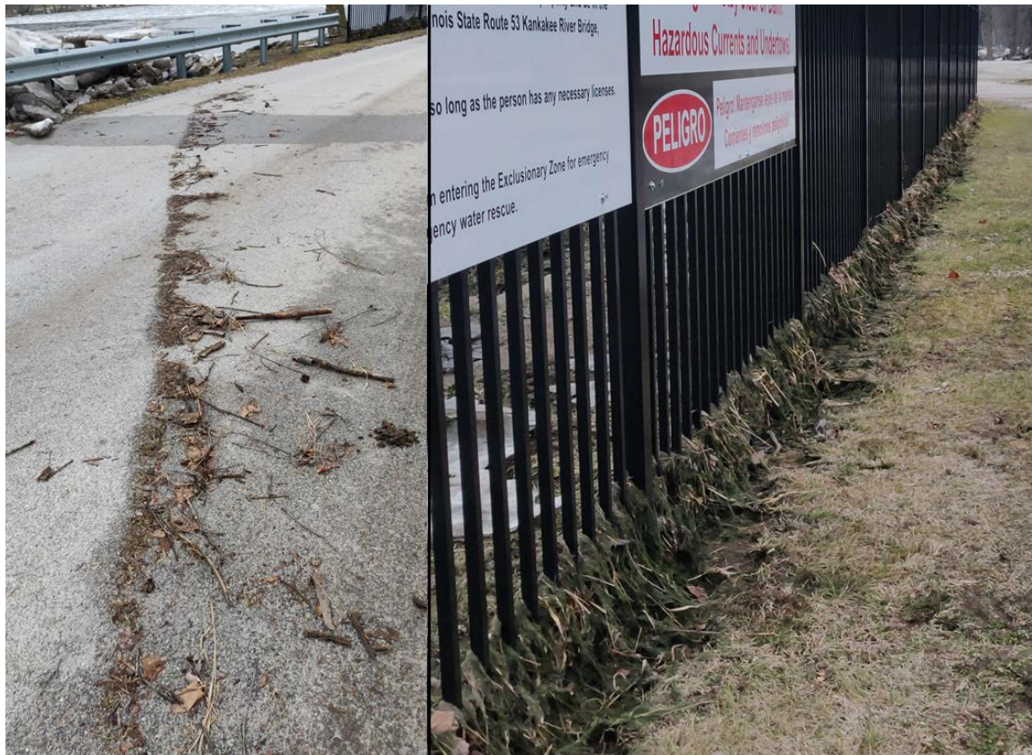
Figure 12. Vegetation debris lines on the roadway in Island Park and vegetation stuck in the fence near Wilmington Dam visible on January 30. These high water marks suggest a peak water level of about 539 feet elevation.
