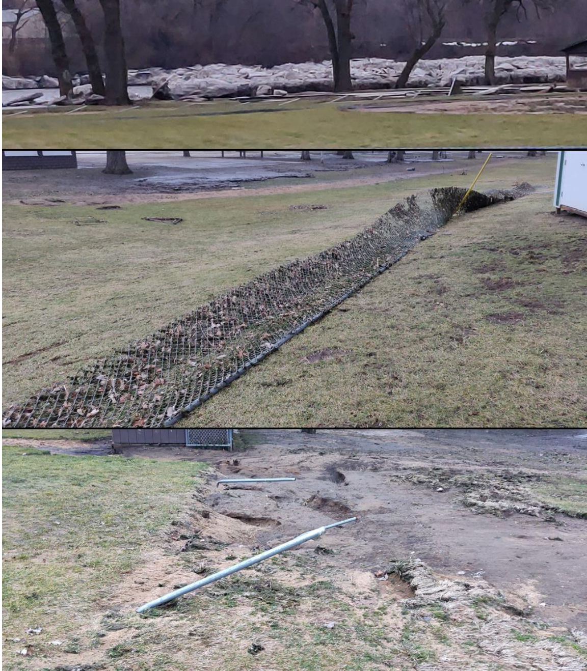
Figure 14. Chain link fencing damaged at the north (downstream) end of Island Park in Wilmington due to flooding and ice flows. Photographed on January 30.
