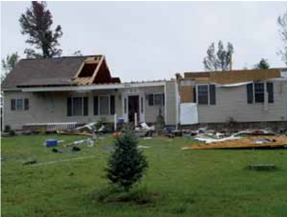
Damage from the Stokesdale tornado and a 79 mph downburst wind gust at the Raleigh-Durham International Airport during the passage of the remnants of Hurricane Ivan. September 17, 2004, Guilford County Emergency Management, Stokesdale Fire Department, Doug Schneider, Darin Figurskey and Jeff Orrock.
