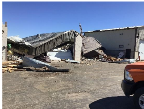
Damage to a KDOT facility in Sharon Springs.
