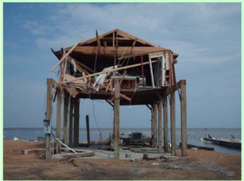
Damage from surge Caplen, Texas on the Bolivar Peninsula
