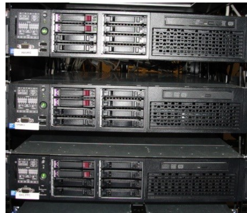
Photo above is the AWIPS servers.
