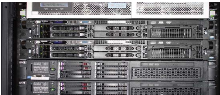
New AWIPS servers at the Peachtree City Weather Forecast Office
