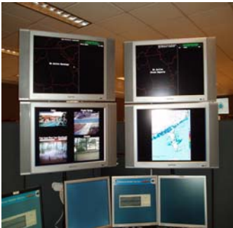
Four large LCD monitors used for situational awareness at one of the Warning Forecaster desks.
