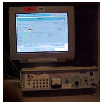
The NOAA Weather Radio Console Replacement System which creates "the voice" and broadcasts to 16 transmitters.
