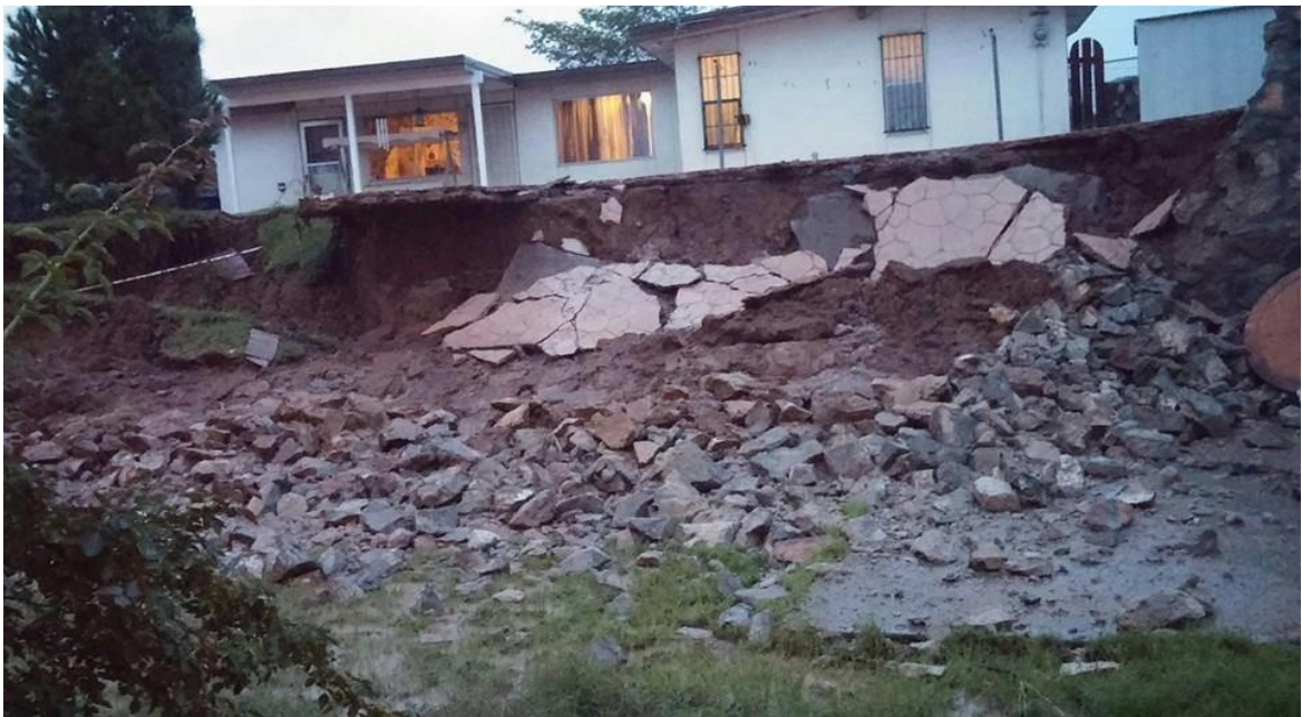
September 22 heavy rains and flooding severely damaged portions of northeast El Paso.
