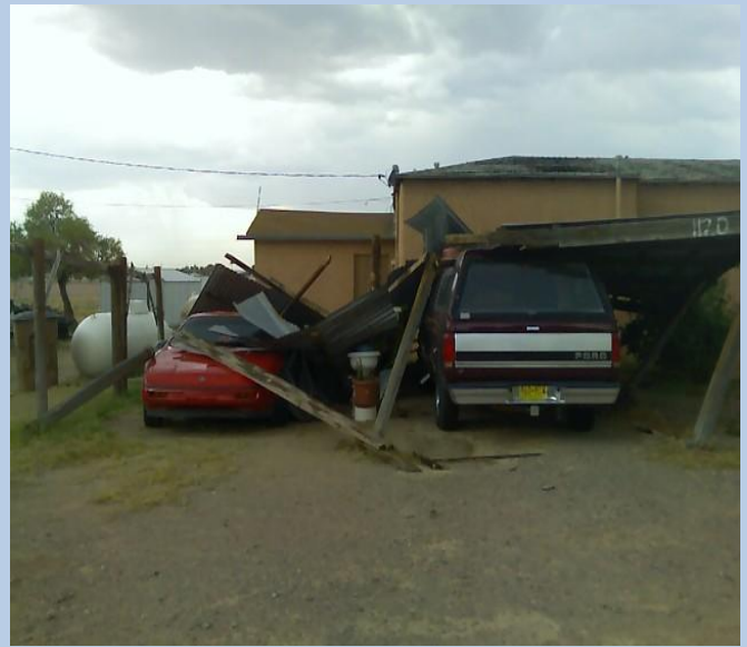
July 10 thunderstorm winds damage this carport in Las Cruces. ( Anna Bishop)
