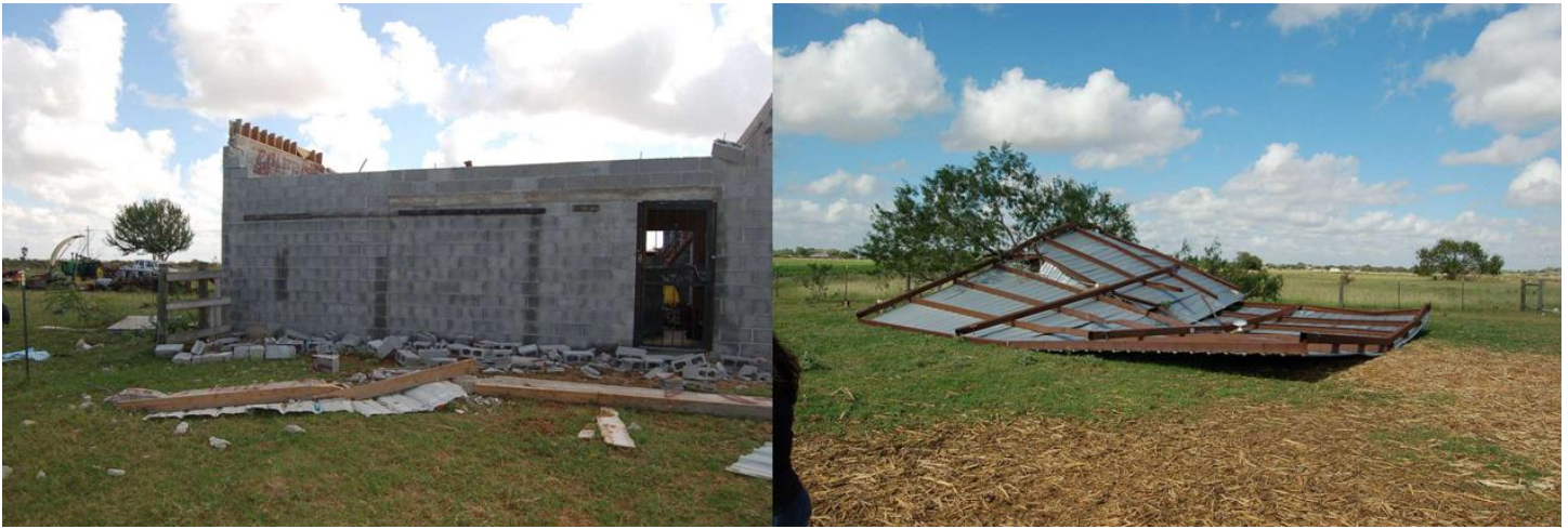
Damage to cinderblock storage building after metal roof was lifted by thunderstorm winds at approximately 617 PM on October 18th, 2012.
