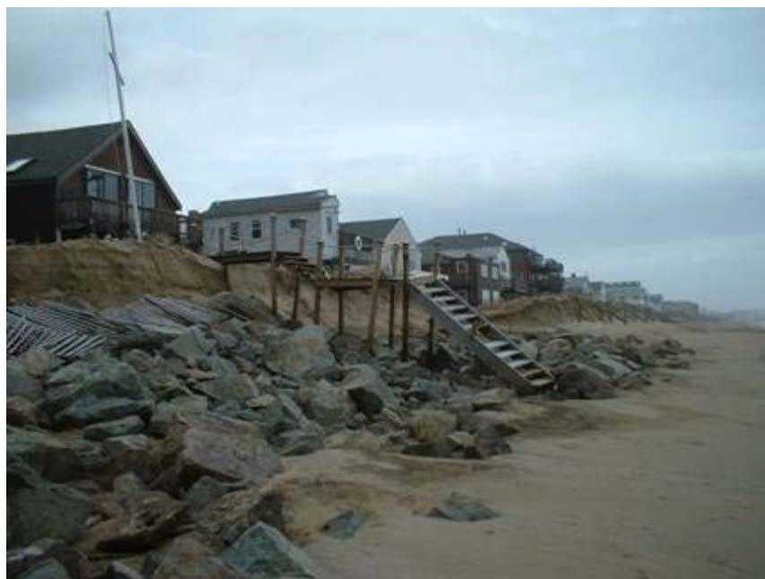
Coastal Flood Damage in Salisbury, MA (Nicole Belk, WFO Taunton Photo)
