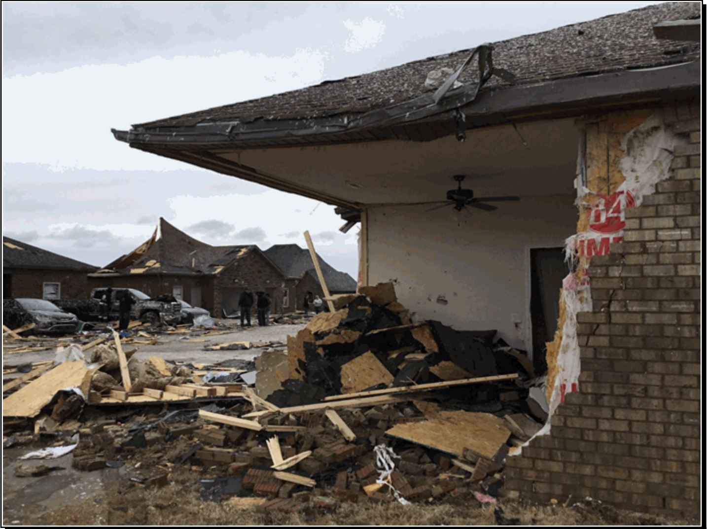
Numerous duplexes on Holland Drive in eastern Clarksville, Tennessee were severely damaged by an EF-2 tornado during the evening of February 24, 2018.
