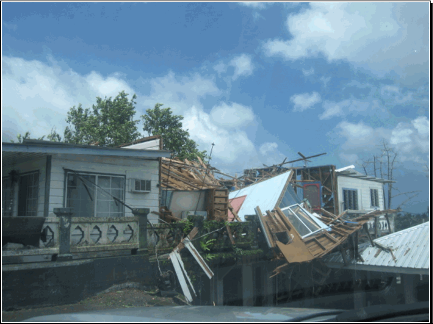
Damaged home in Faleniu from Tropical Storm Gita, American Samoa; Credit: Carol Baqui.
