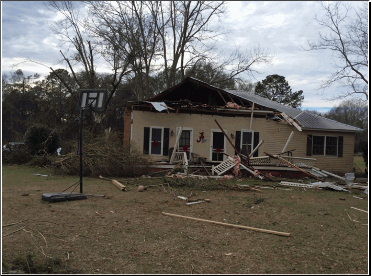
An EF2 intensity tornado produced extensive damage to this home on Gin Creek Road, just east of Luverne, AL.
