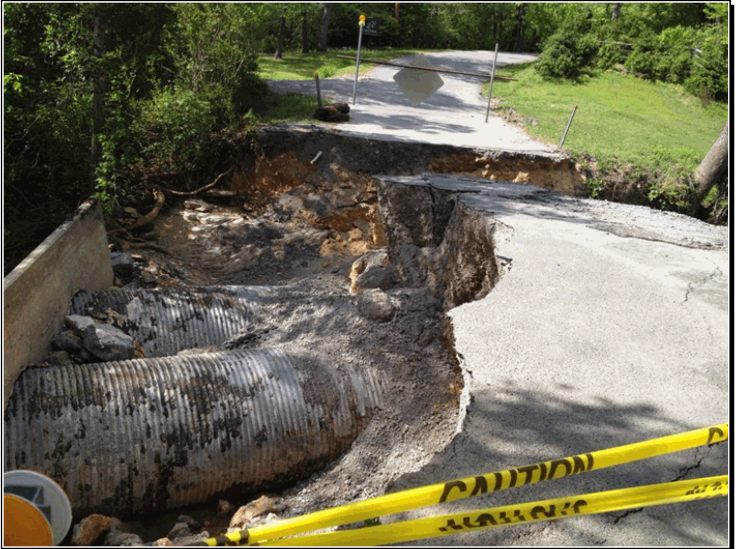
Road washed out between Valley Head and Mentone.
