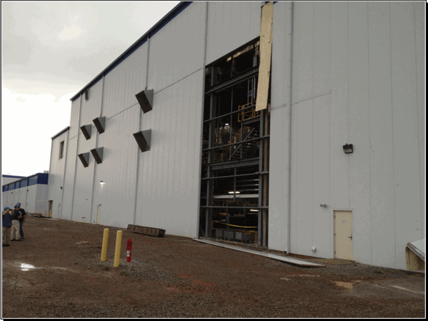
Section of wall blown out at Toray Plant (outside of Decatur) off Hwy 20.
