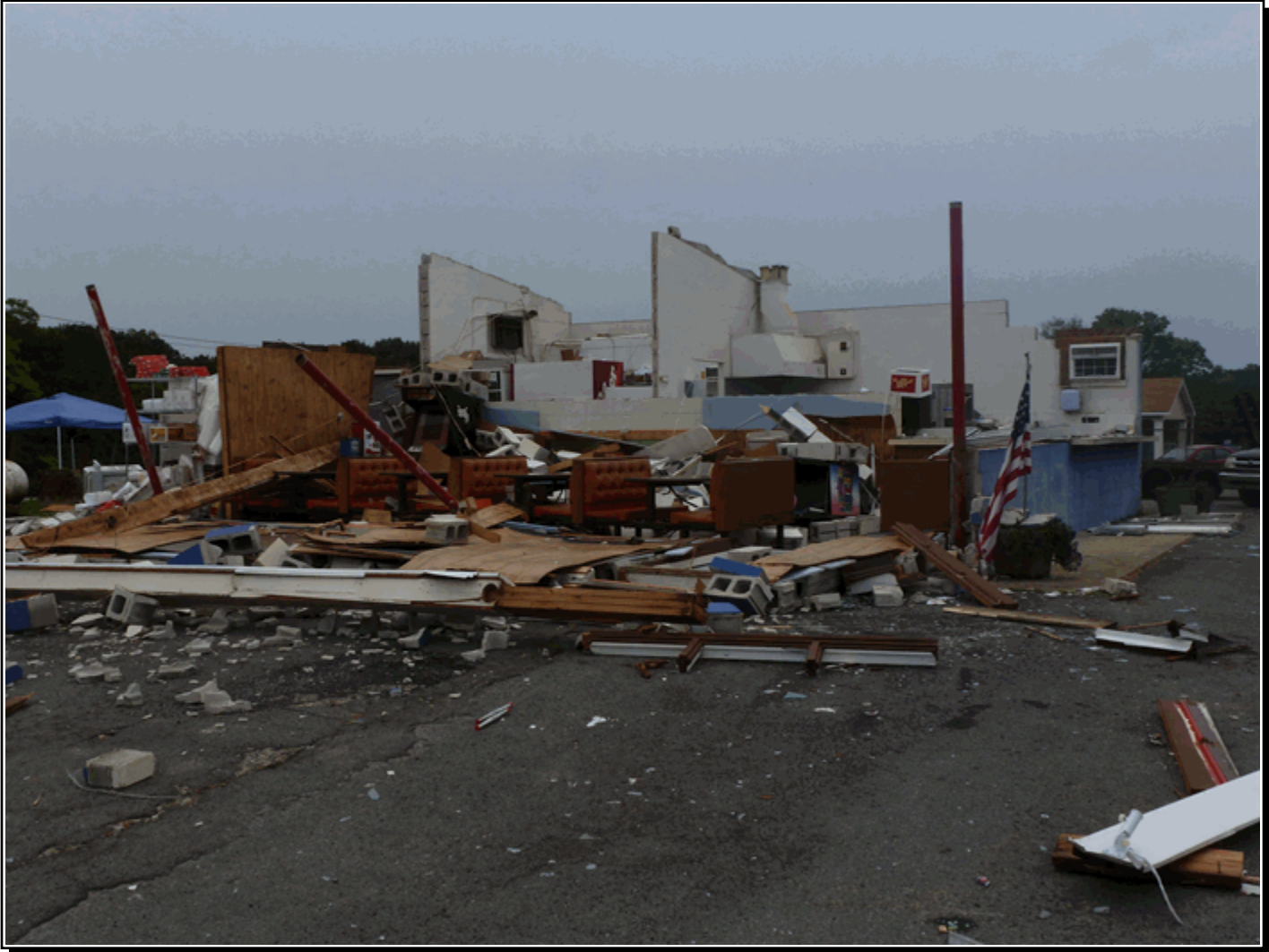
Claysville, Alabama Snack Bar destroyed by a microburst on July 1, 2012. Photo by David Nadler, Warning Coordination Meteorologist, NWS Huntsville, Alabama.
