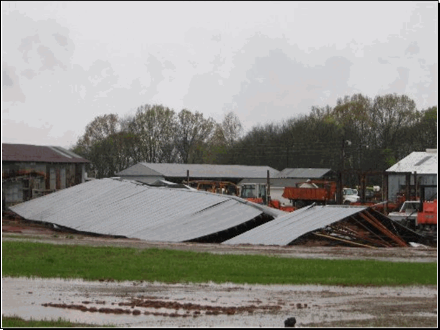
Building flattened at the Colbert County Road Department about 2 miles east of Tuscumbia along Highway 72. This corresponded to EF-1 damage.
