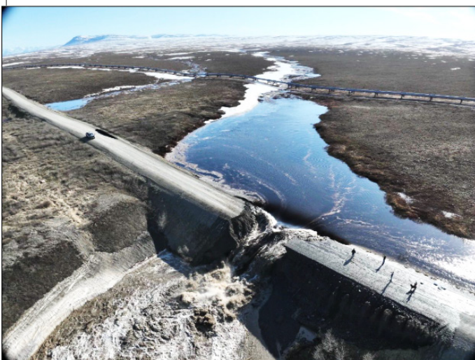
MP 315 washout on the Dalton Highway on June 14th. Image courtesy of AKDOT
