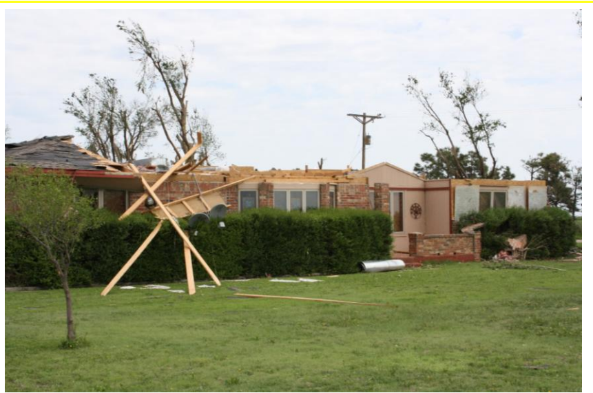
Most of the roof was blown off of a home near Pampa, Texas by a tornado on May 15, 2009.
